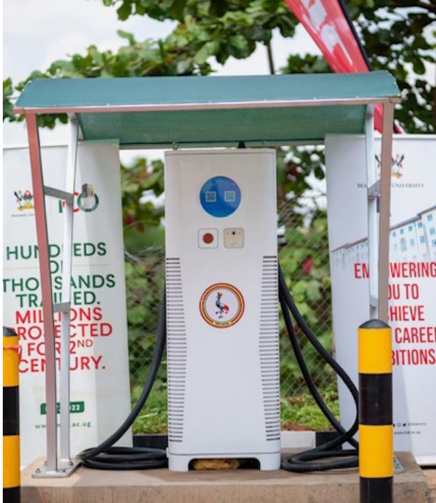
Charging station in Kampala, Uganda. Photo: EFD Mak-Center
